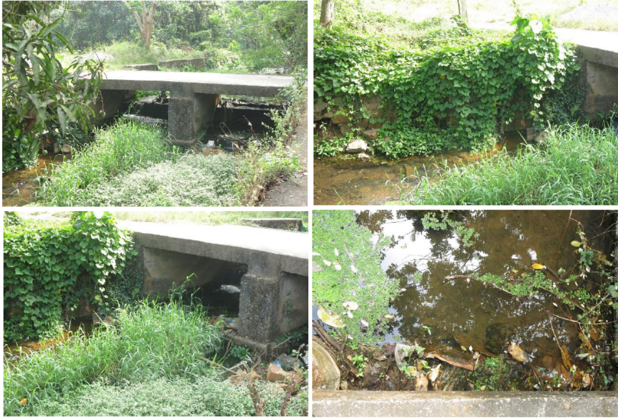
Fig. 2.Choked canal and sluice with weeds.
